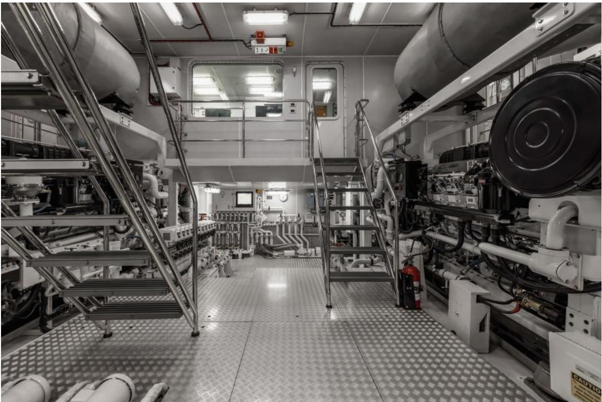
LAUREL 240'/73.15m Delta 2006/2014 Engine Room
