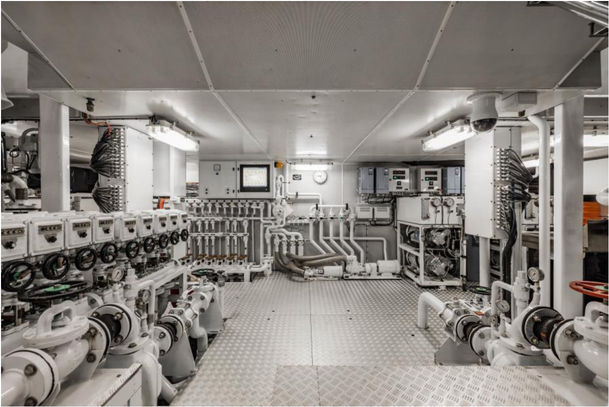
LAUREL 240'/73.15m Delta 2006/2014 Engine Room
