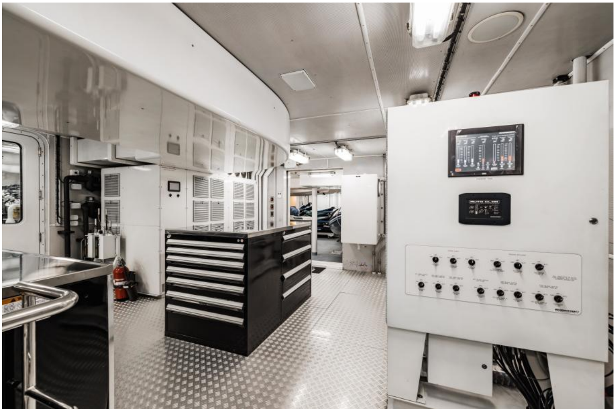
LAUREL 240'/73.15m Delta 2006/2014 Engine Room
